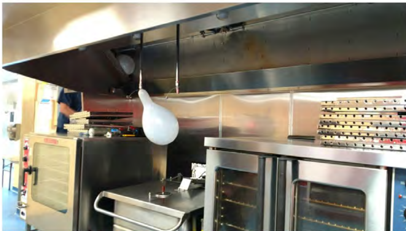
Balloon test on suppression nozzles in progress
